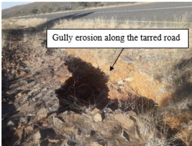
Figure 24: The magnitude of erosion observed along a tarred road going towards Magotlhwane village
